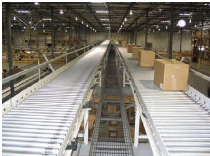
After product is packed (see below), it travels by conveyor to a sliding shoe sortation system.
